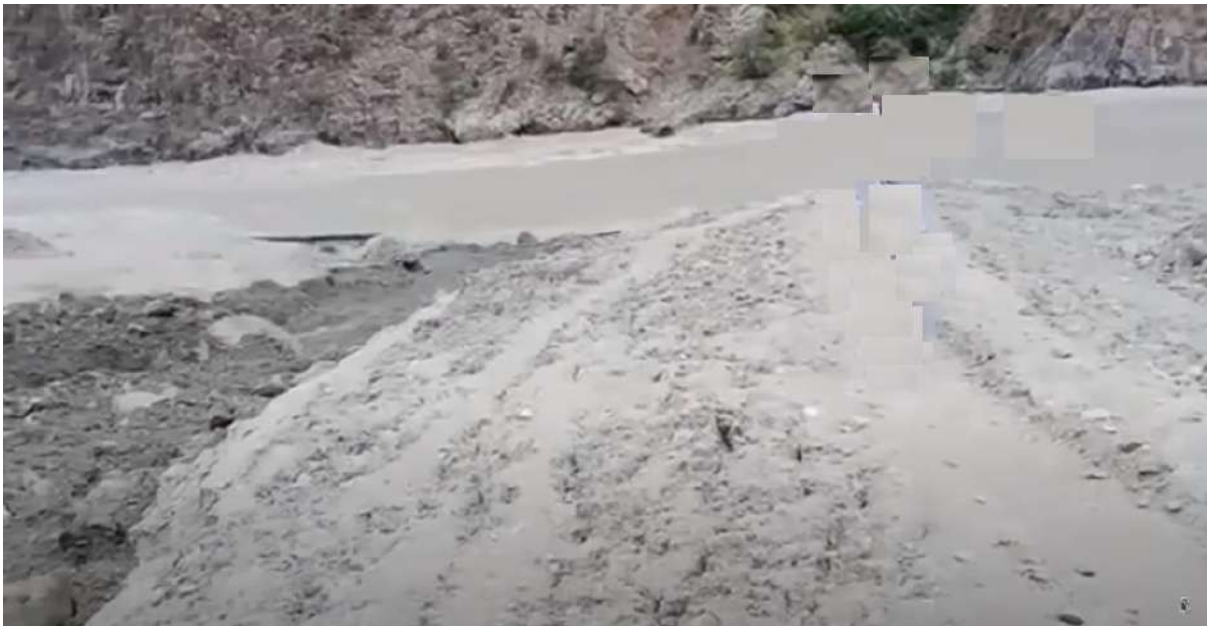
Figure 14: Frame-11, Sinking bridge, barely visible
