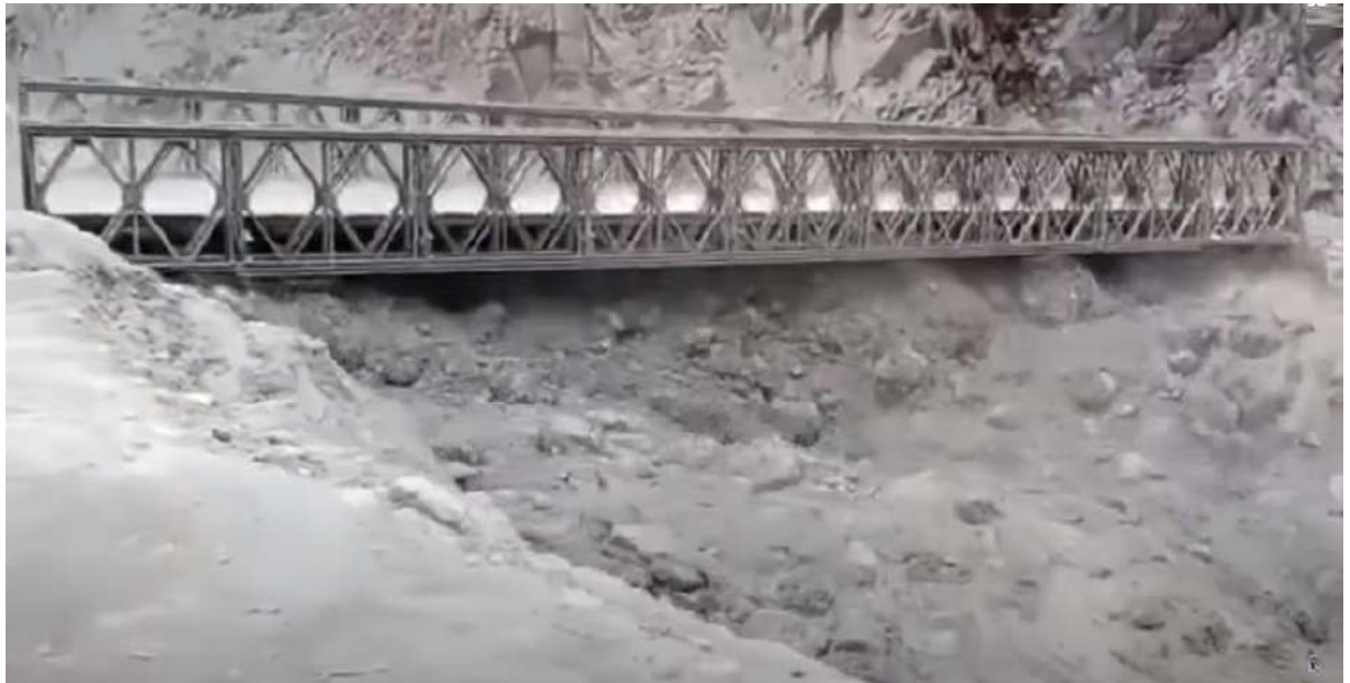
Figure 10: Frame-7, Bridge quite far away from the original position and has almost completely lost its support
