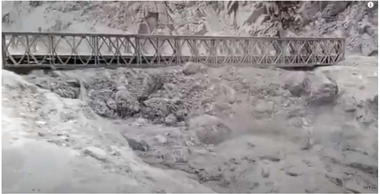
Figure 8: frame-5, Bridge moves still farther away from the original position and sitting on debris
