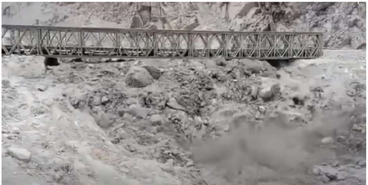
Figure 7: Frame-4, Bridge moves farther away from the original position and sitting on debris
