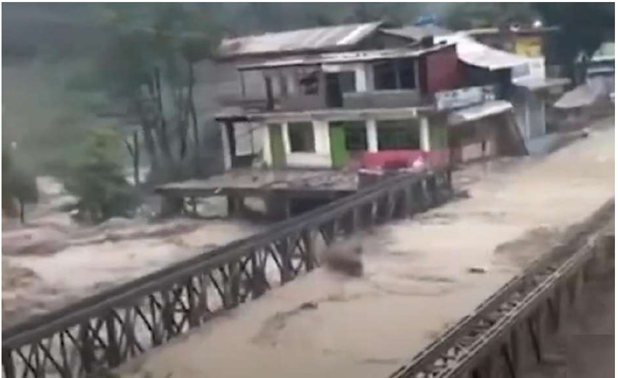
Figure 4: Frame-1, Frame-1, Water flowing across the deck
