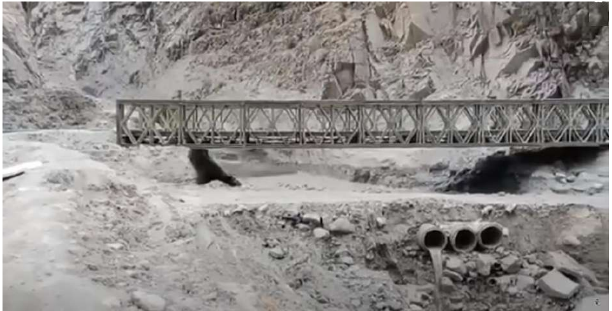
Figure 5: Frame-2, Bridge dislocated from its abutment
