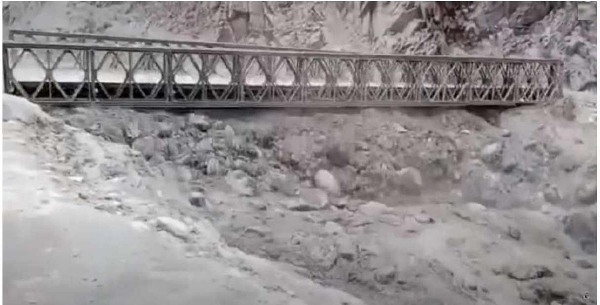
Figure 9: Frame-6, Bridge very far away from the original position and about to lose its support from debris
