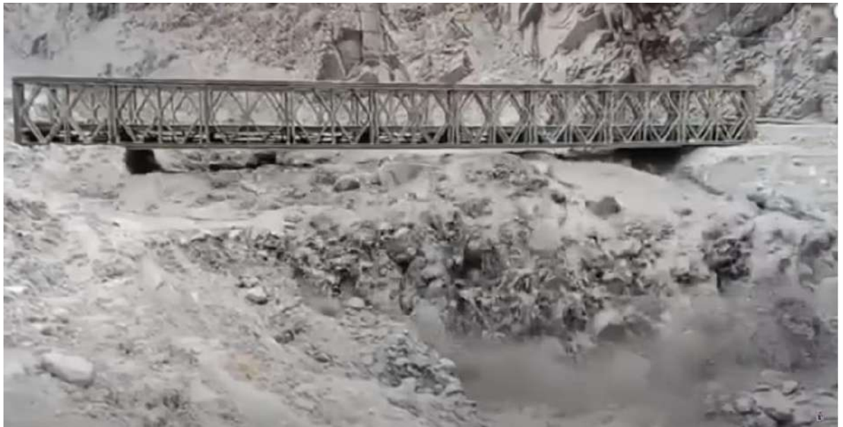
Figure 6: Frame-3, Bridge adrift
