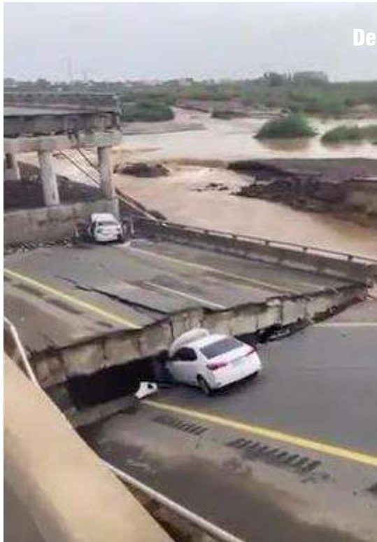
FIGURE 5: TURN IN THE STREAM CENTERLINE, COLLAPSED DECKS AND VEHICLE IMPACT
