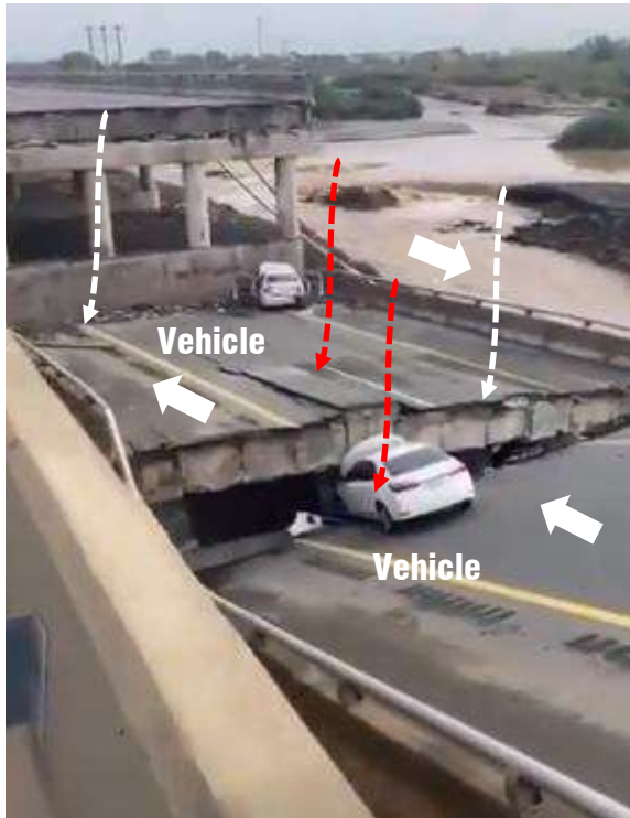
FIGURE 9: FINAL AND ORIGINAL POSITIONS OF COLLAPSED DECK SYSTEM
