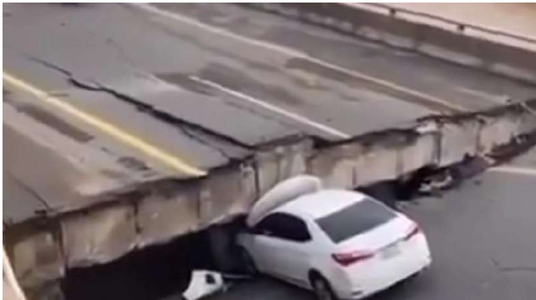
FIGURE 10: BADLY DAMAGED DECK OF THE COLLAPSED SPAN
