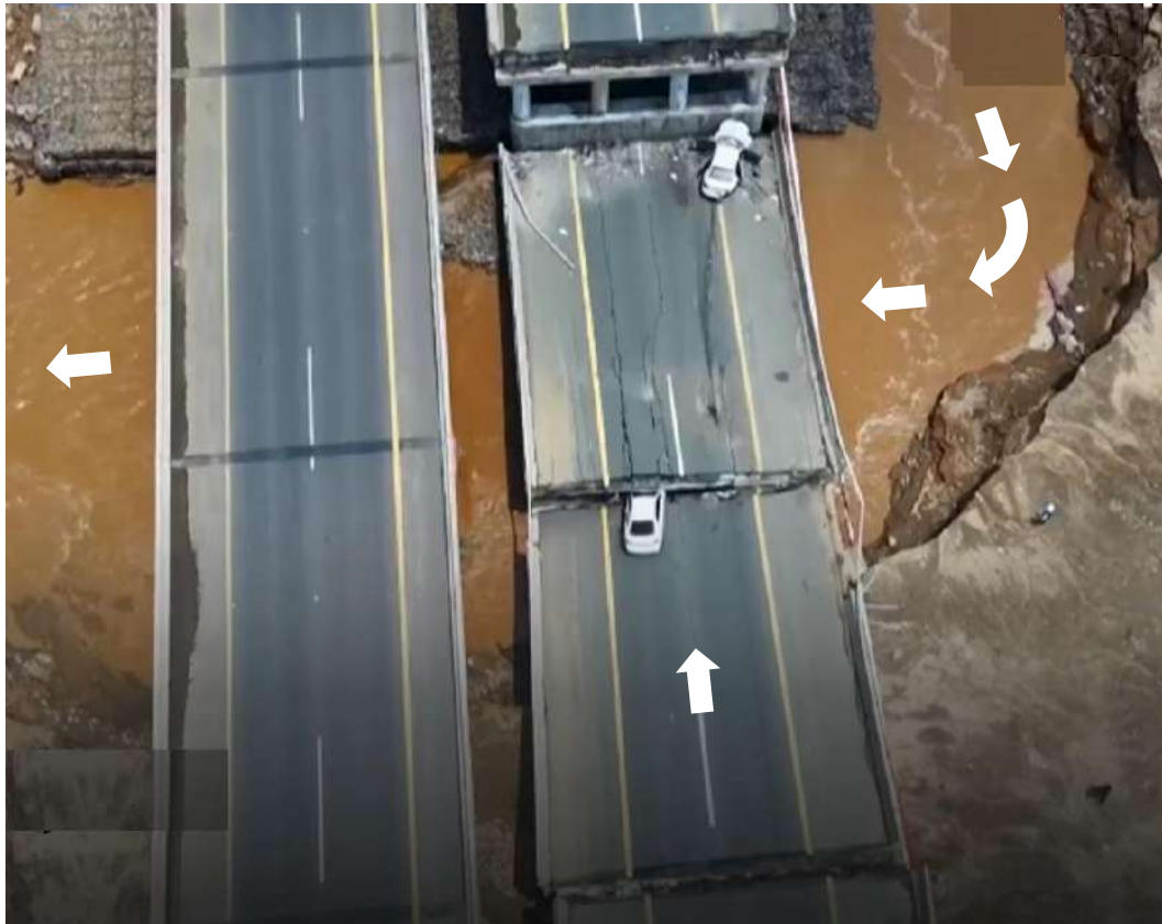
FIGURE 3: AN AERIAL CLOSE-UP OF THE COLLAPSED DECKS SHOWING DAMAGED VEHICLES AND THE DECKS
