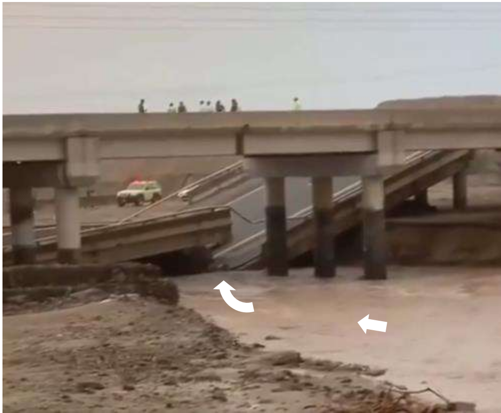
FIGURE 7: AN ELEVATION VIEW OF THE COLLAPSED DECKS
