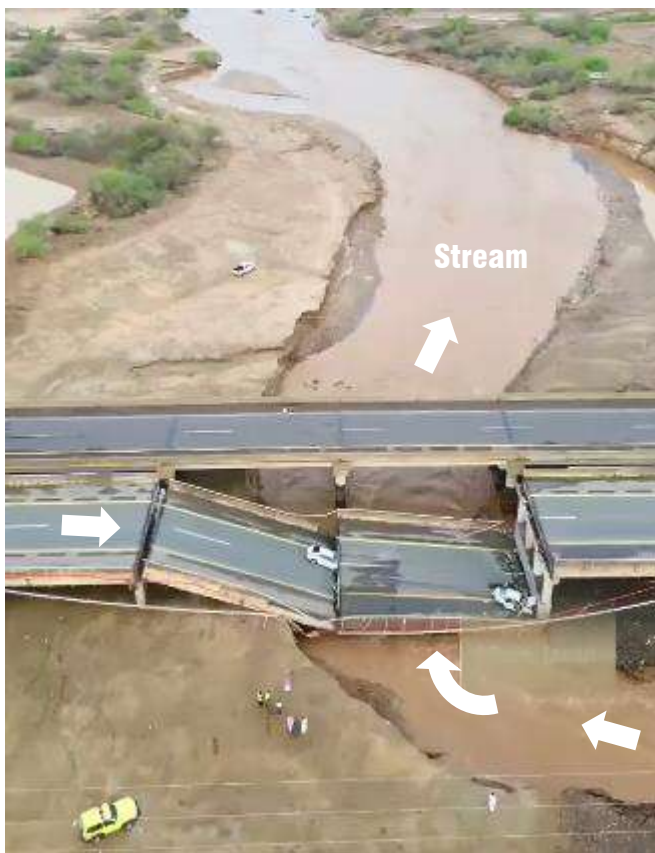
FIGURE 6: AN AERIAL VIEW OF THE COLLAPSE BRIDGE
